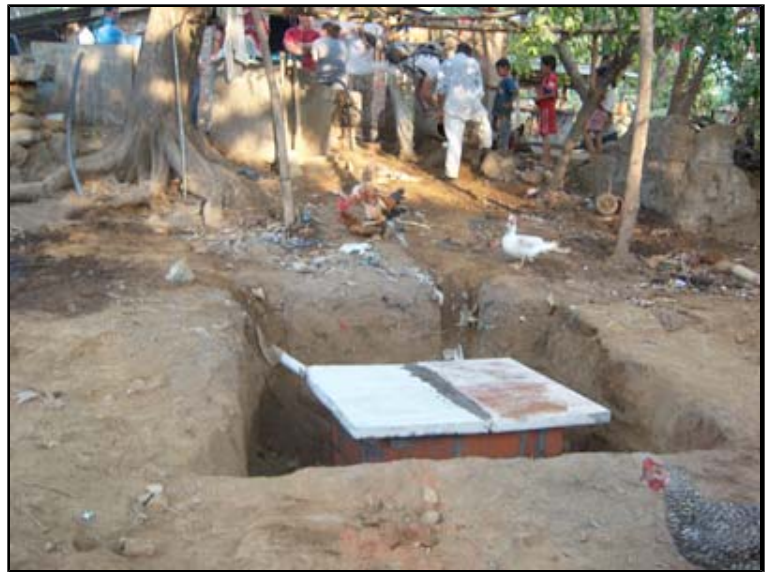
Two concrete panels cover a brick seepage pit built by the students behind one of the villager's homes. The pit will prevent runoff and erosion caused by water used for washing, which will instead be absorbed by the ground.
